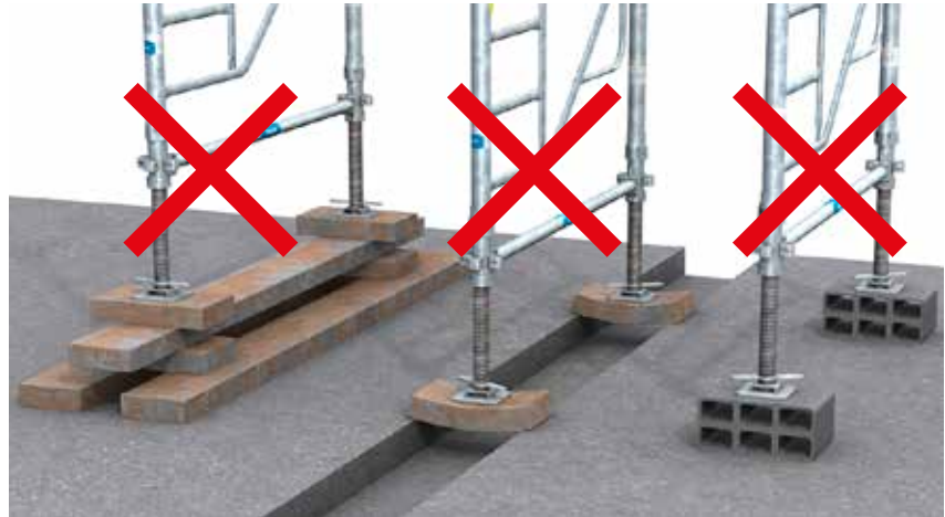
Excessive chock stacking
